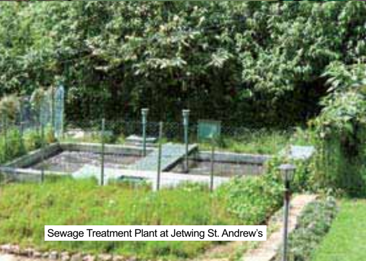
Treated sewage water ready for use
